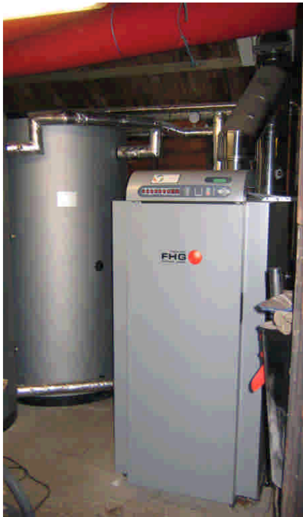
Figure 3: Froling 70 kW log boiler and accumulator tank (left).
