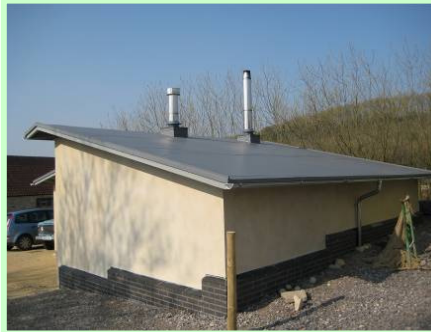
The boiler house. The right hand flue comes from the pellet boiler (the left hand flue comes from the LPG back up).
