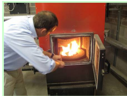
Philip Niemand clears ash from the combustion chamber.
