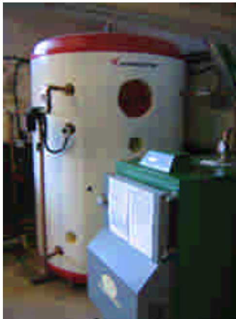
Figure 2: Vigas 40kW log boiler and accumulator tank (left).
