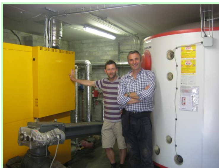
Tim Reed of Tredethick Farm Cottages and Kevin Lindegaard of Crops for Energy with the Tredethick Boiler
