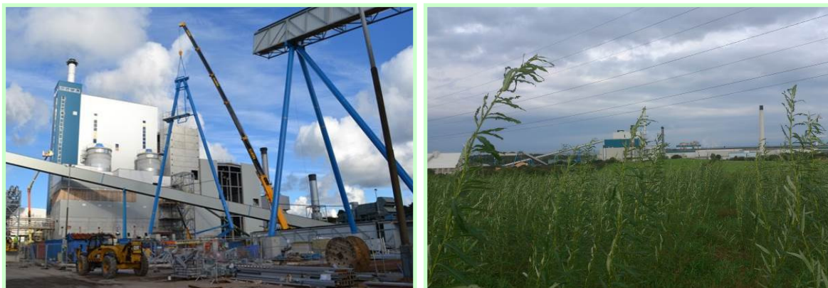
Left: Construction of the 50 MW biomass CHP plant (Image courtesy of Iggesund).
