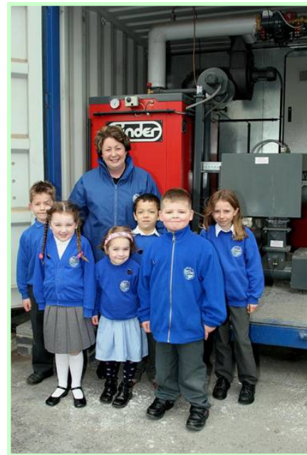
The biomass boiler at Dunham on Trent Primary School is supplied with SRC woodchip by Strawson's Energy. The SRC crop is situated at Manor House Farm, East Drayton less than 1 mile away. (Image courtesy of Farmers' Weekly)
