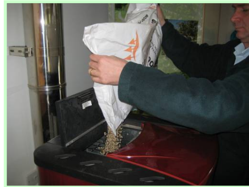
Adding wood pellets to the integral hopper. This needs to be done 1-2 times per day.
